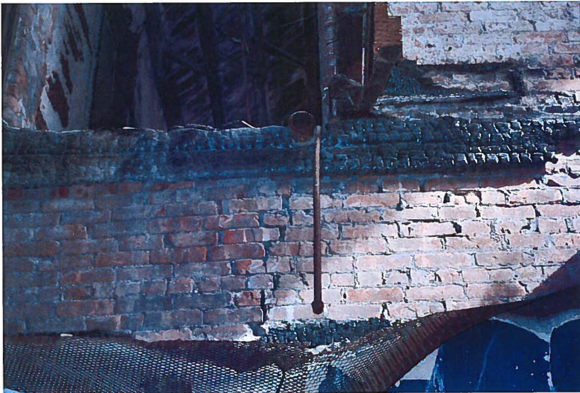
Additional fire damage to second floor
