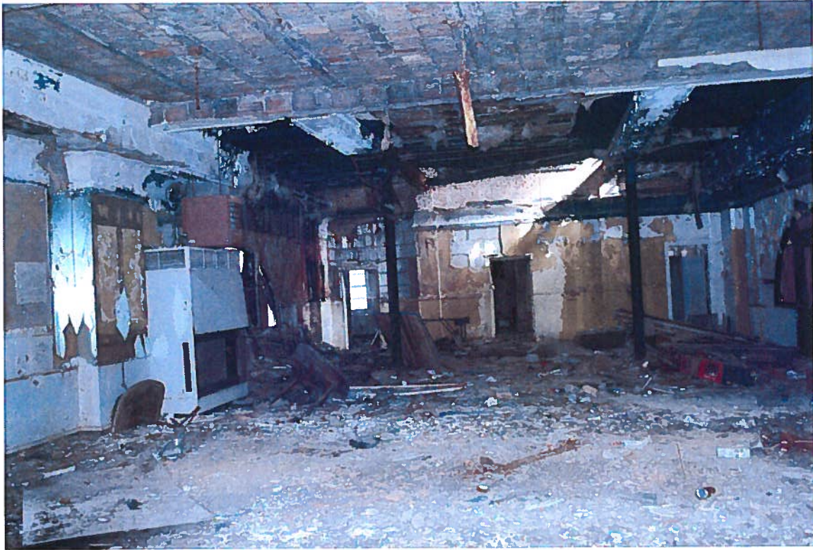
First floor deterioration
