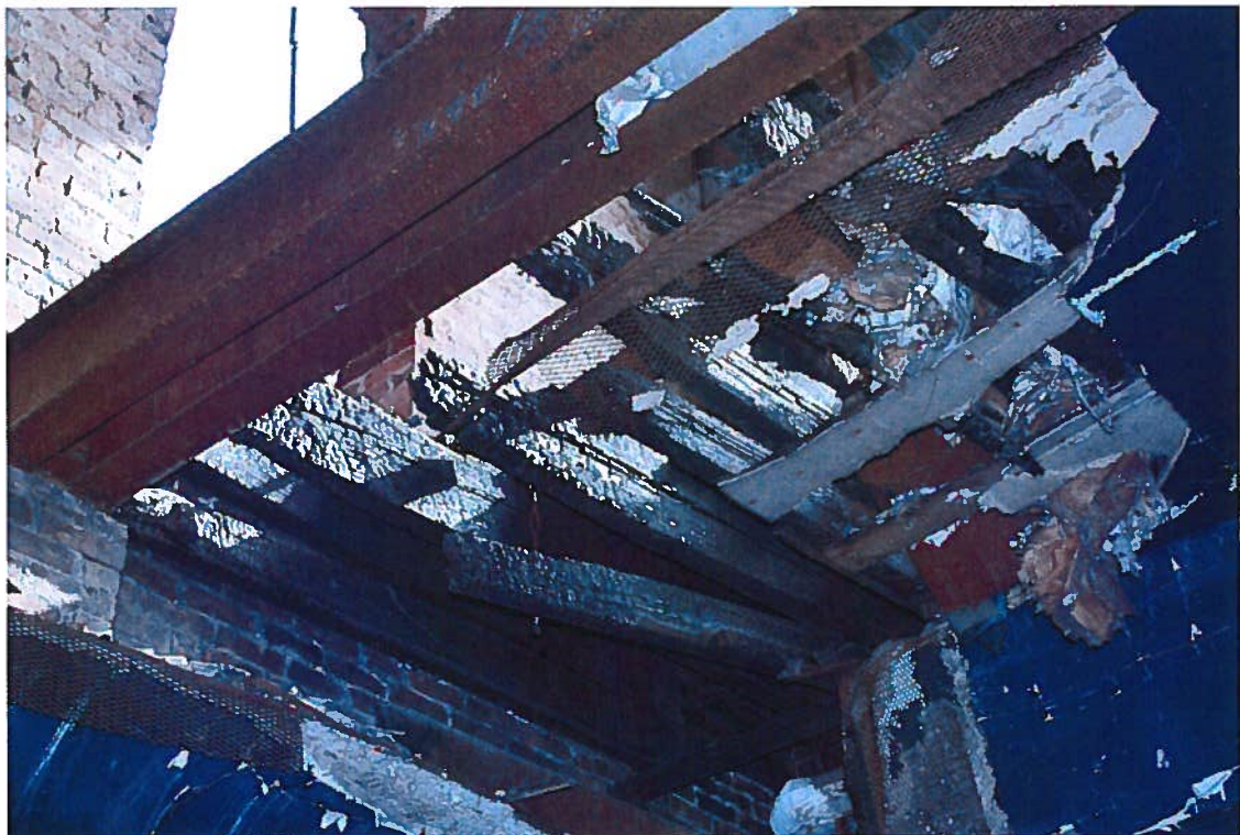
Fire damage on 2 nd floor near north tower
