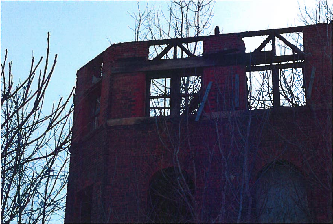
Deterioration and missing roof on north tower.
