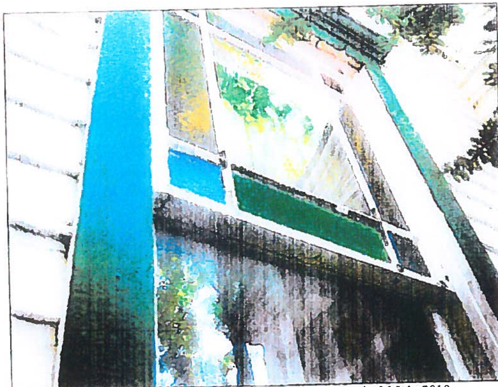
Photo 40: Mapes House damaged sash and glazing in need of repair. 06 July 2010
