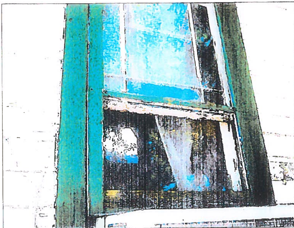
Photo 62: Mapes House Exterior paint chipped or missing North sides-window sash and siding 06 July 2010
