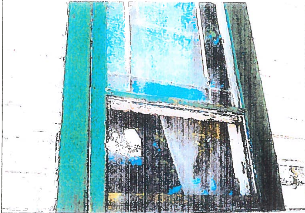
Photo 39: Mapes House damaged sash and glazing in need of repair. 06 July 2010
